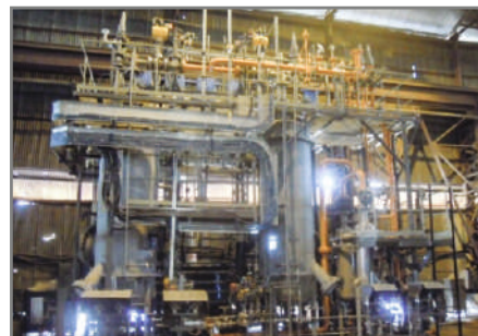
Ethylene dryer for Opal- Dahej
