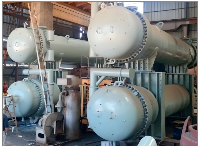
Stacked Heat Exchangers - TKIS - NRL Numaligarh
