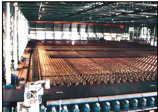
Cooling Bed 60 Mtr x 80 Mtrs with roller tables for Welsupn Anjar for Plate Mill Project
